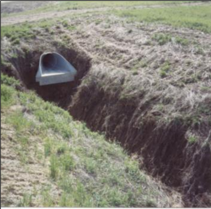
Erosion in Gräben
